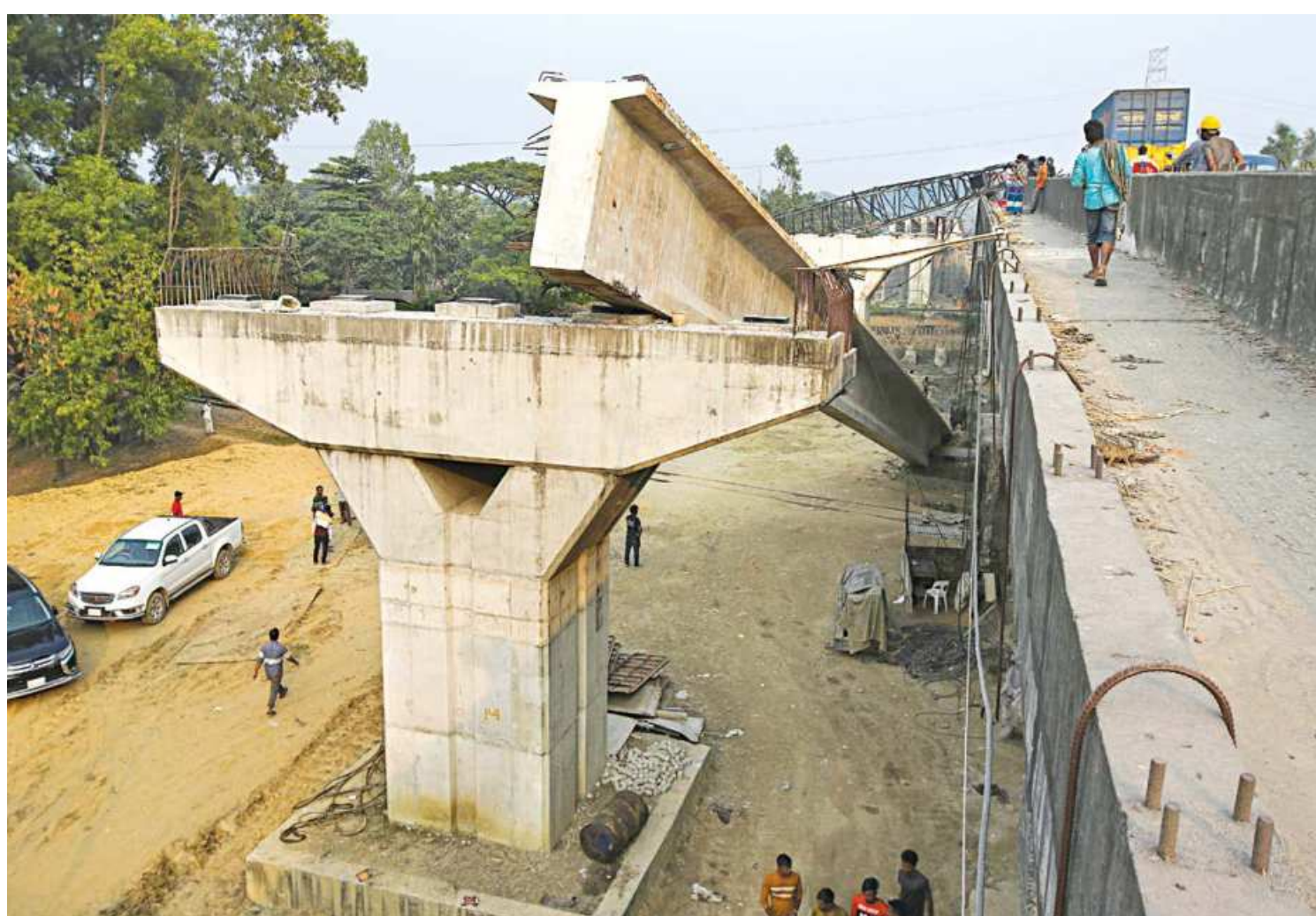
The massive girder of an under-construction overpass in Chattogram's Bayezid-Foujdarhat Link Road area is precariously propped against a pillar. The wire of a crane that was used to lift the girder had snapped yesterday, causing the part of the concrete and steel structure to fall on a truck and injuring one of its occupants, who was admitted to a local hospital.
