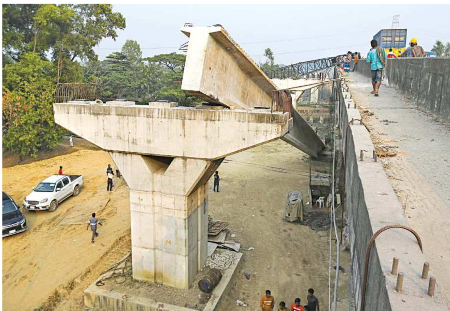
The massive girder of an under-construction overpass in Chattogram's Bayezid-Foujdarhat Link Road area is precariously propped against a pillar. The wire of a crane that was used to lift the girder had snapped yesterday, causing the part of the concrete and steel structure to fall on a truck and injuring one of its occupants, who was admitted to a local hospital.
