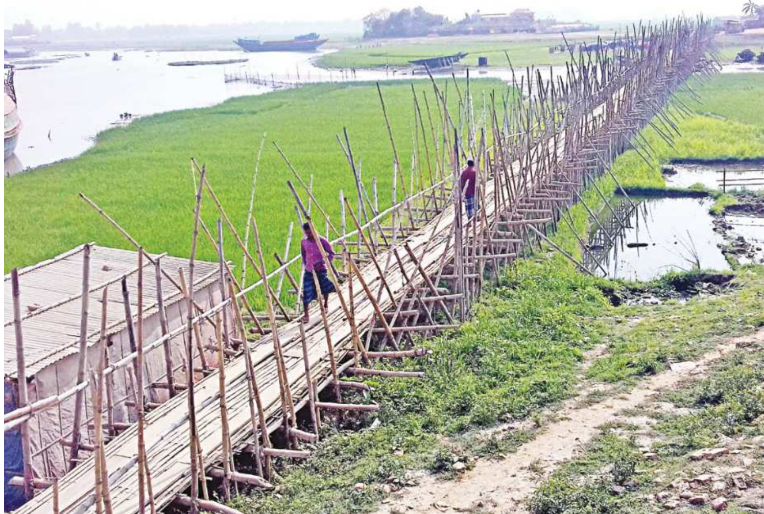
Over one lakh people of 15 villages in Aruail and Pakshimul unions of Brahmanbaria's Sarail depend on this six-foot wide bamboo bridge over the Chetra River. Their only other option is to use boats, but that too becomes impossible in winter. A proper bridge would hugely benefit the residents of the area.
