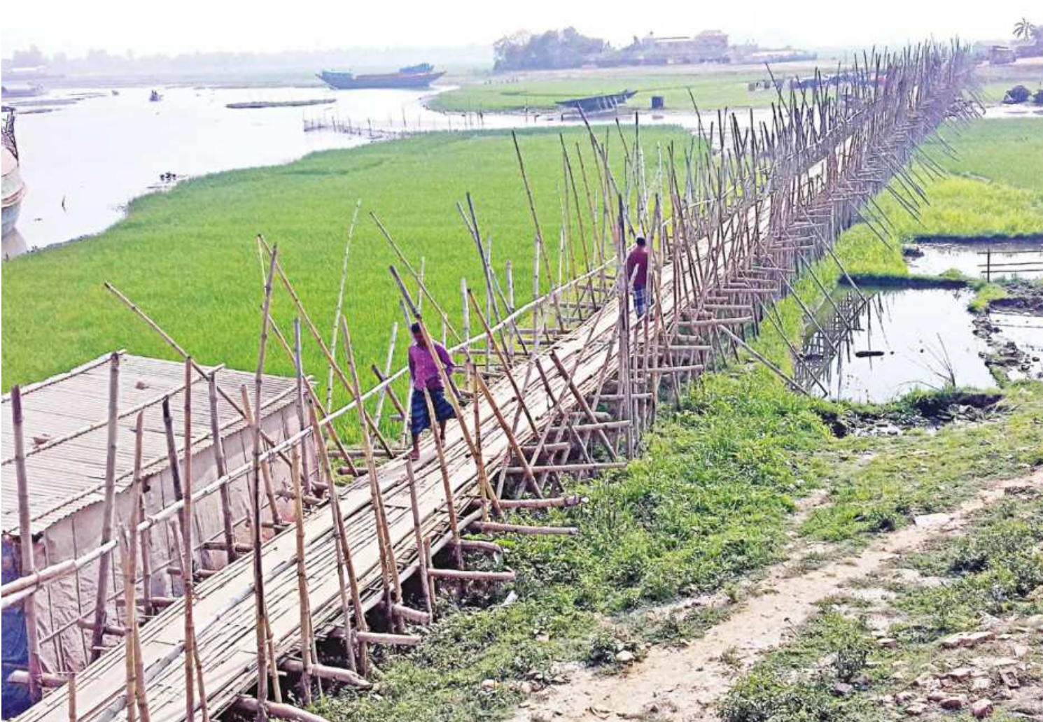
Over one lakh people of 15 villages in Aruail and Pakshimul unions of Brahmanbaria's Sarail depend on this six-foot wide bamboo bridge over the Chetra River. Their only other option is to use boats, but that too becomes impossible in winter. A proper bridge would hugely benefit the residents of the area.
