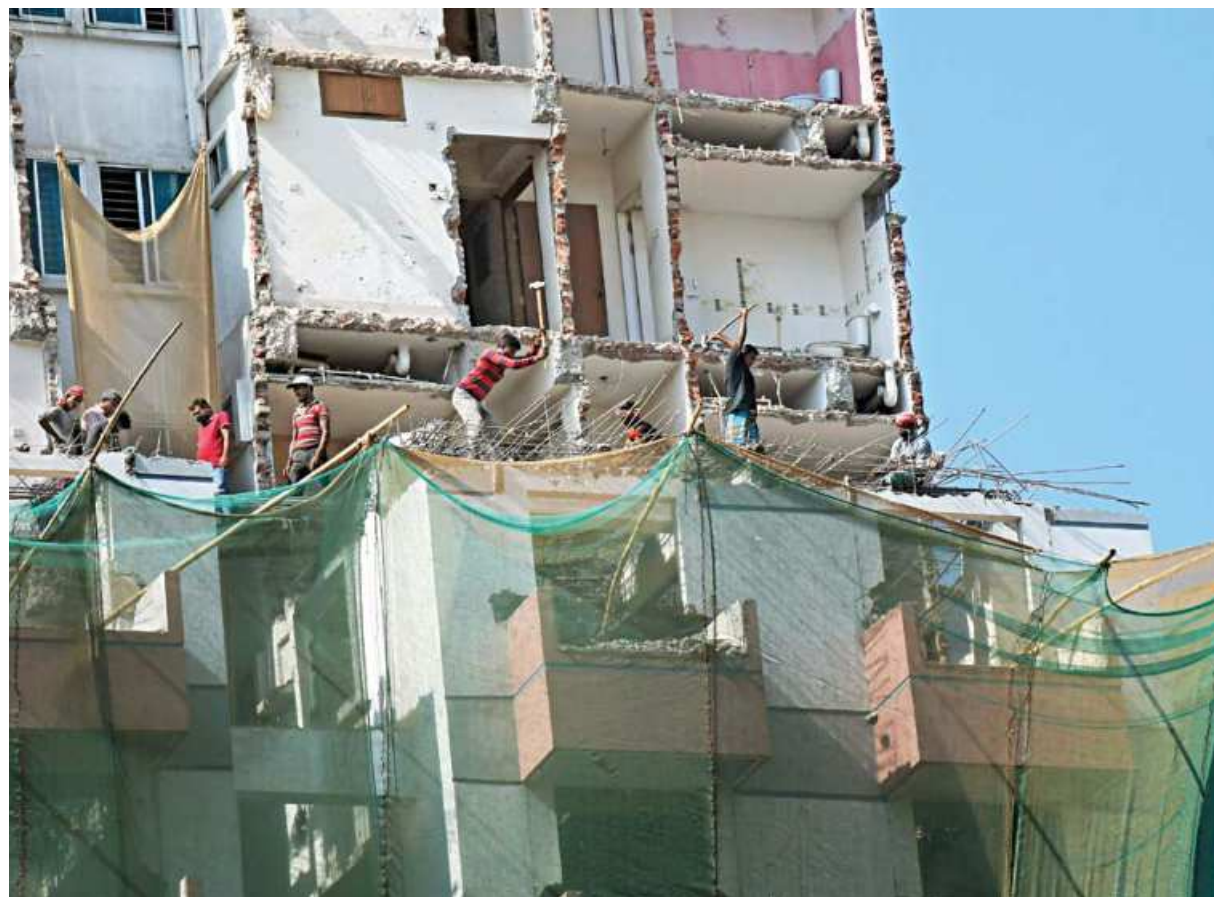
Workers without any safety gear demolishing a part of a building in Tejgaon rail crossing area yesterday. Such disregard for safety often results in fatal accidents.
