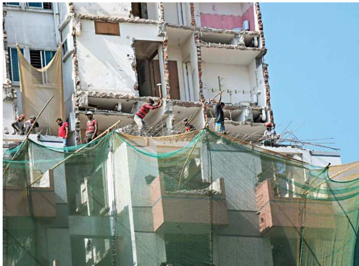
Workers without any safety gear demolishing a part of a building in Tejjao rail crossing area yesterday. Such disregard for safety often results in fatal accidents.
