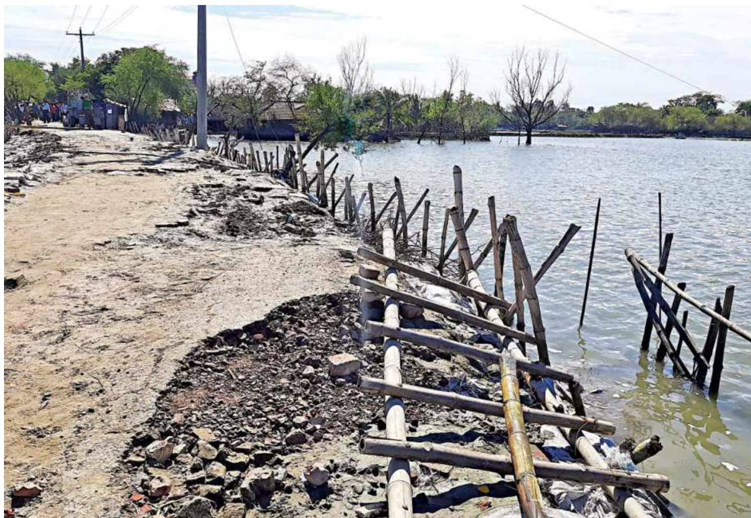
This road in Prapatnagar union of Satkhira's Assasuni upazila has been badly damaged for about six months since Cyclone Amphan hit the area in May, causing hardships for local people. A large area of the union is still submerged due to entry of water through some breaches in the Kopotakho and Kholpetua river embankments.
