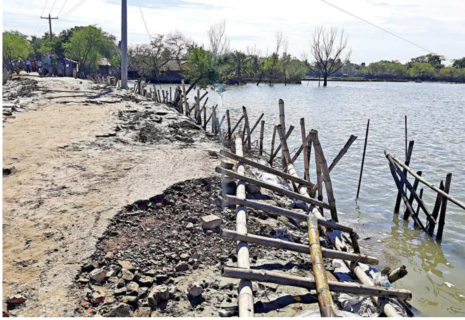
This road in Prapatnagar union of Satkhira's Assasuni upazila has been badly damaged for about six months since Cyclone Amphan hit the area in May, causing hardships for local people. A large area of the union is still submerged due to entry of water through some breaches in the Kopotakho and Kholpetua river embankments.
