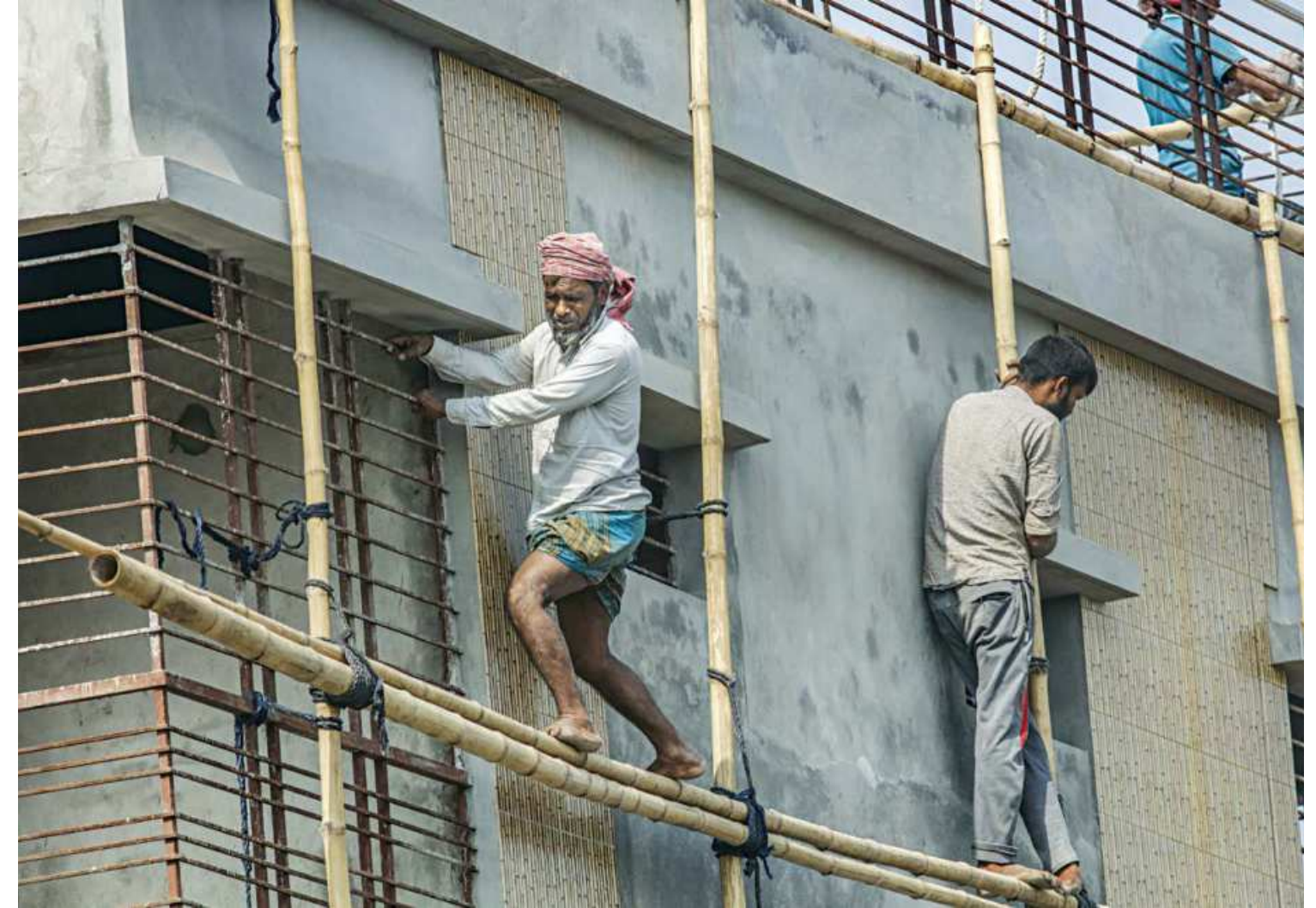
Construction workers working on a high-rise building without any safety gear, ultimately risking their lives, in Mohammadpur's Tikkapara area. The photo was taken yesterday. PHOTO: RASHED SHUMON
