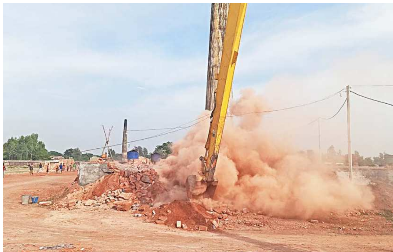
Five acres of land was reclaimed after Bangladesh Inland Water Transport Authority conducted a drive yesterday to remove illegal structures at Ferihat area of Narayanganj's Sadar upazila, on the bank of Dhaleshwari River. Such drives will continue, as per the High Court's directive, officials said.
