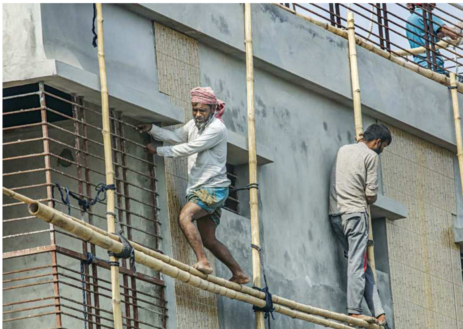
Construction workers working on a high-rise building without any safety gear, ultimately risking their lives, in Mohammadpur's Tikkapara area. The photo was taken yesterday.
