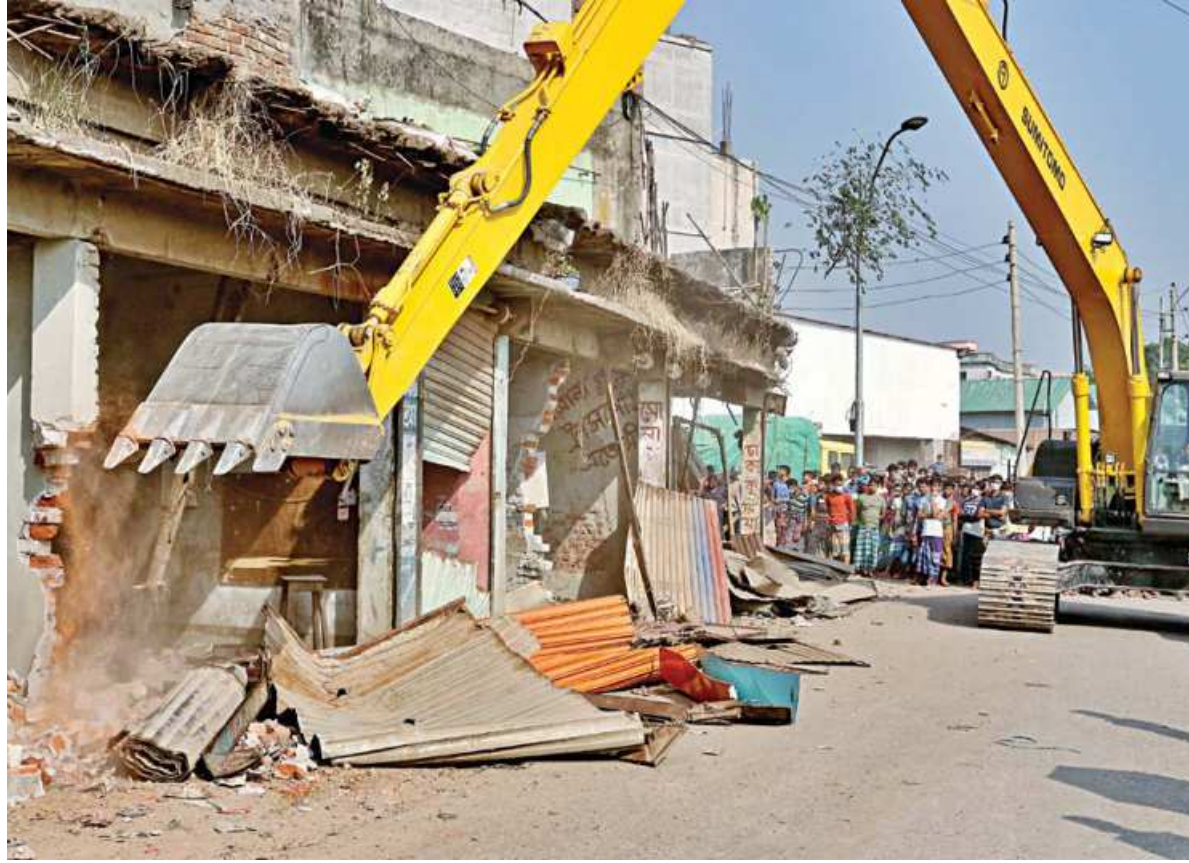
An excavator of Bangladesh Inland Water Transport Authority (BIWTA) knocks down an illegal structure built grabbing the Buriganga river in the capital's Shoari Ghat area. The BIWTA continued the drive for the second day yesterday.
