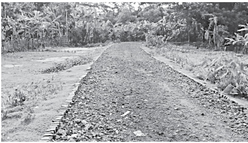
People suffer a lot as construction work of the road at Hoglabuniya village in Pirojpur's Indurkani upazila remains suspended for the last few months due to fund crisis.
