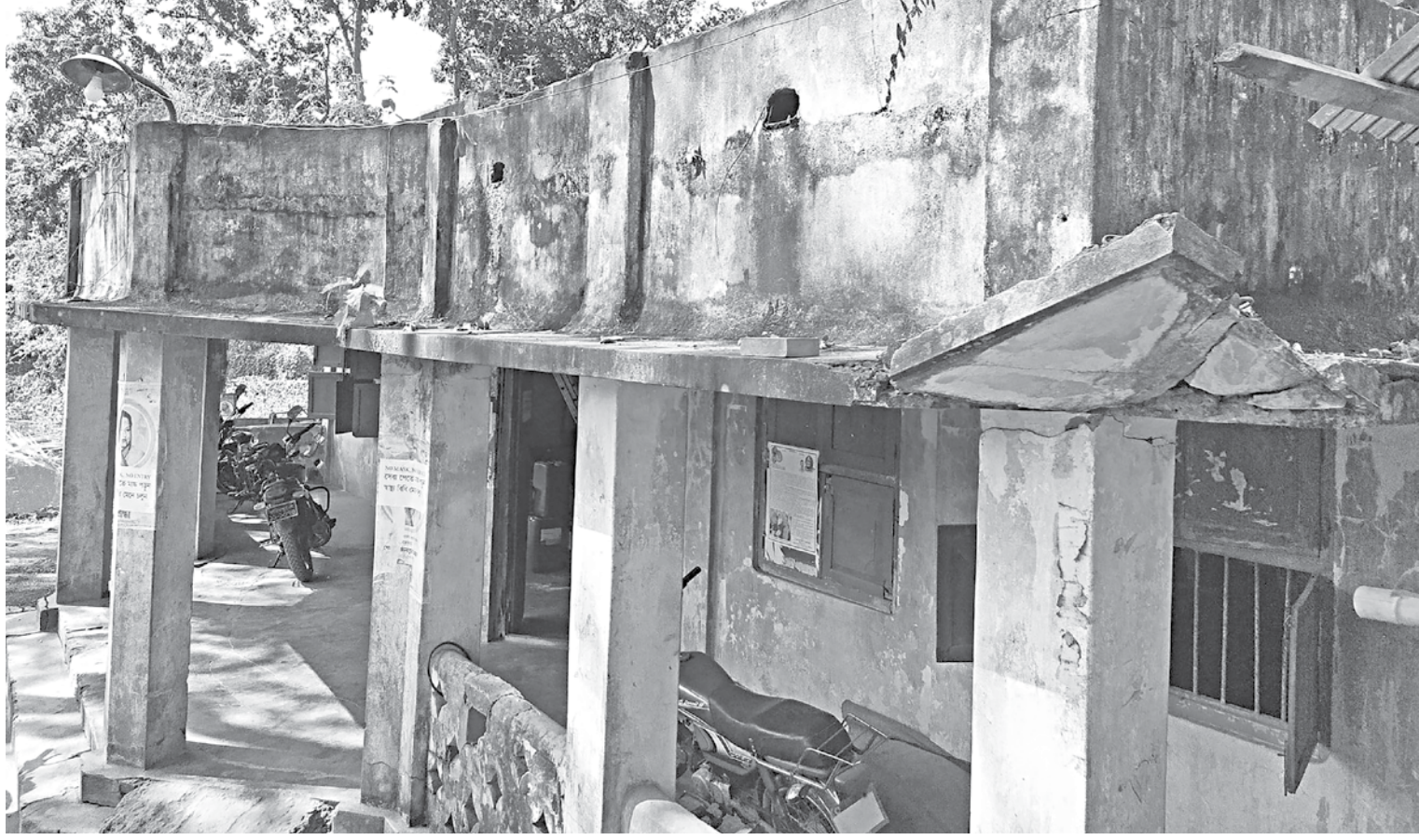
Employees of Nagarkanda municipality in Faridpur has been working in the risky rented building for years amid risk. Below, plaster came off the ceiling of the old building.
