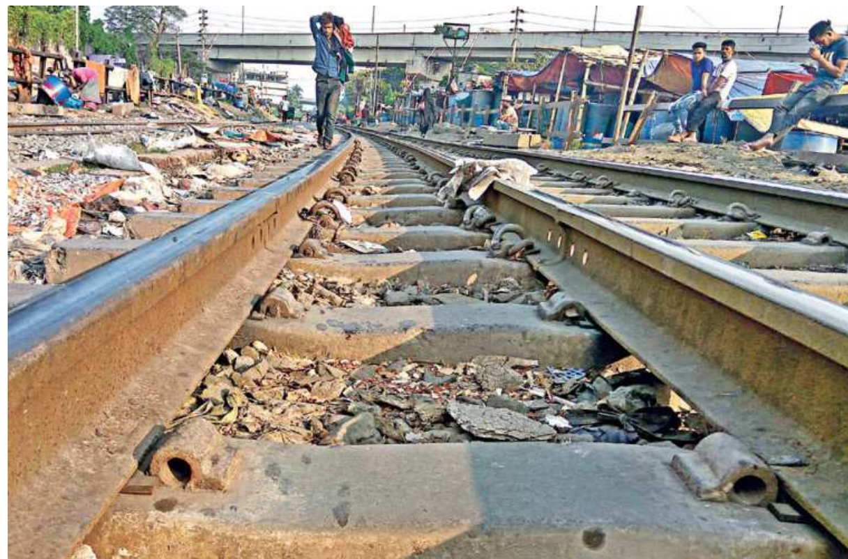
During a walk along the rail line from Malibagh Rail Gate to Tejgaon, this photojournalist found hundreds of sleeper clips -- that hold together the rails and the sleepers of the track -- either broken or completely missing. These clips pose serious risks to trains plying the lines, as political activists have in the past removed clips to derail trains and sabotage rail communication. The photo was taken yesterday.
