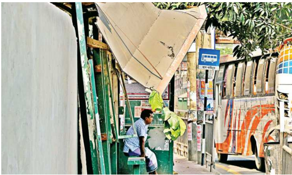
This shabby passenger shed in the capital's Basabo area is on the verge of collapse. The structure poses risk to pedestrians as part of its damaged roof is obstructing their movement. Locals said the shed was set up about a year ago, but no repair work was carried out since then.
