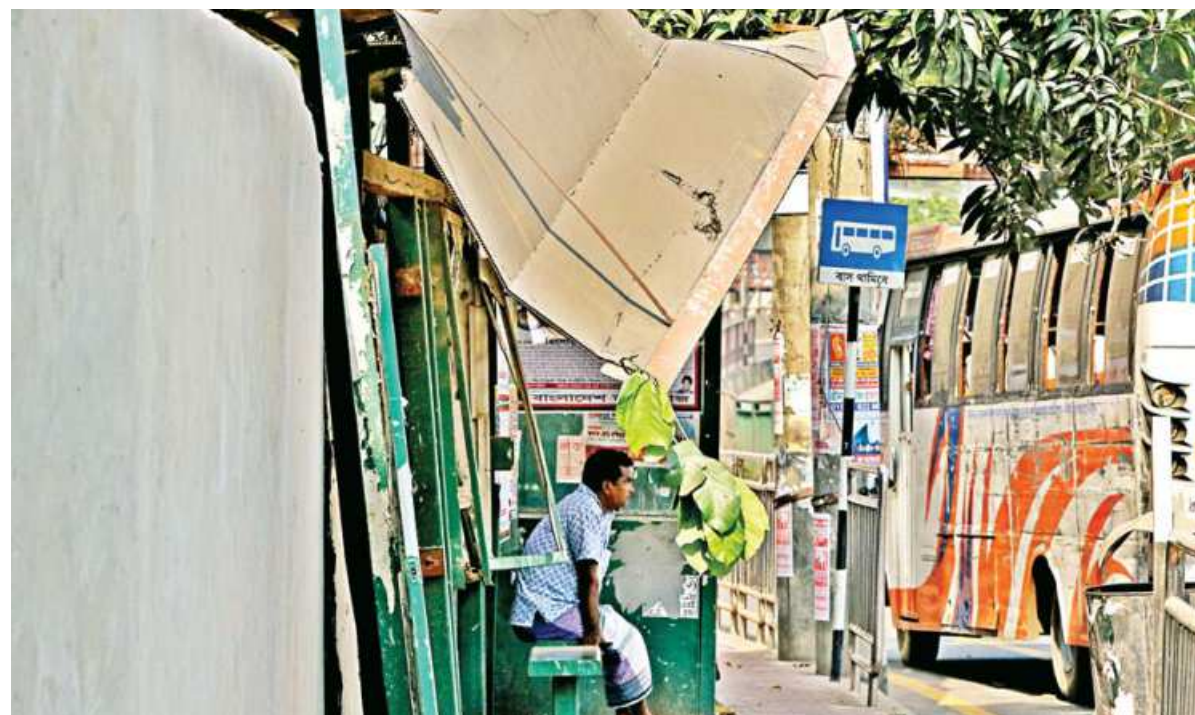
This shabby passenger shed in the capital's Basabo area is on the verge of collapse. The structure poses risk to pedestrians as part of its damaged roof is obstructing their movement. Locals said the shed was set up about a year ago, but no repair work was carried out since then.
