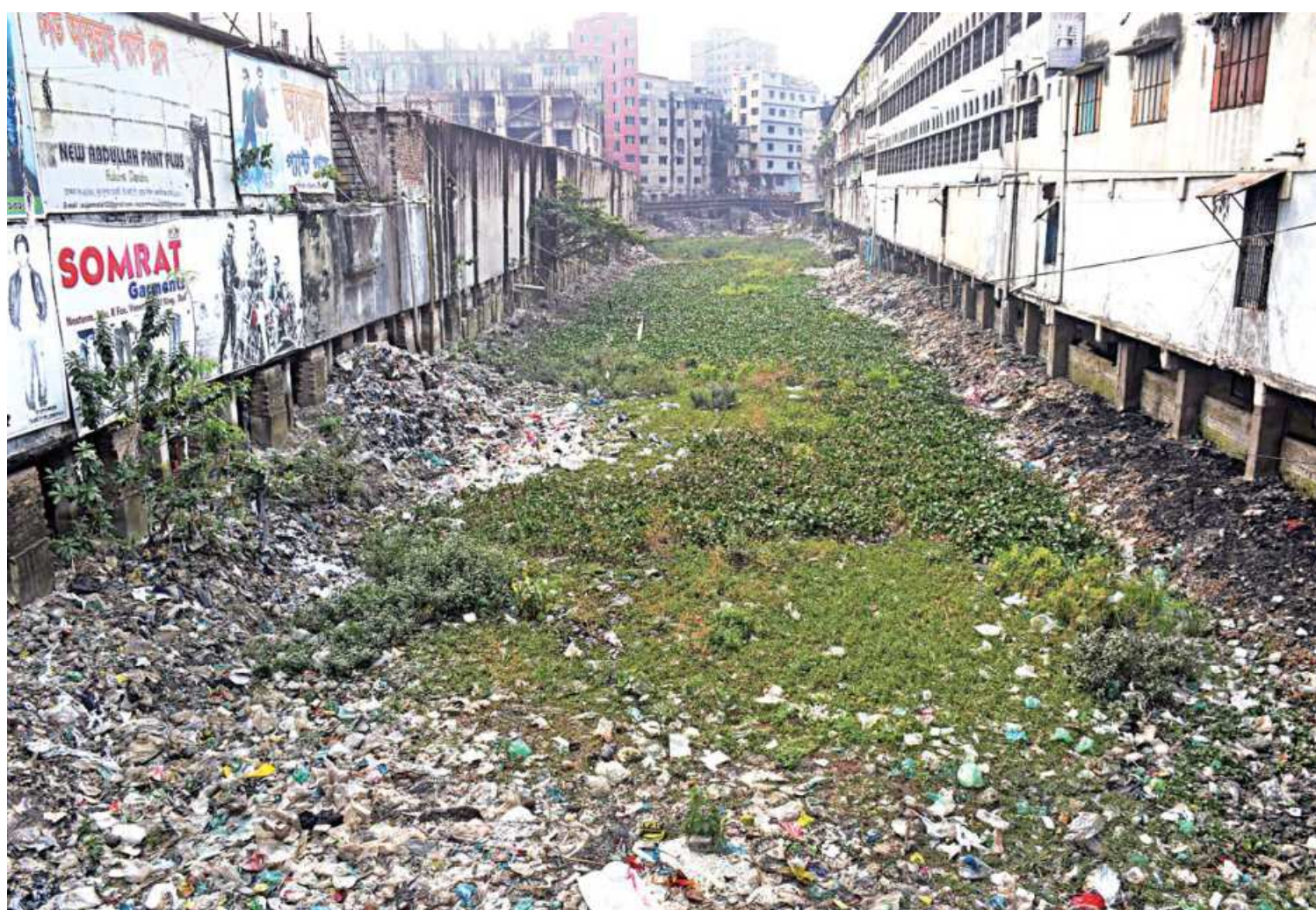
The Shuvadya canal in Keraniganj -- which connects the Dhaleshwari and Buriganga rivers -- is in a sorry state and all but dried up due to dumping of waste from small garment factories in the area. This photo was taken yesterday.
