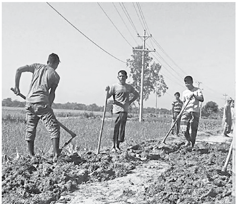
A few of the villagers, young and old, who joined hands to repair the two-kilometre-long dirt road in Shukurullahgaon village of Moulvibazar's Kamalganj upazila.
