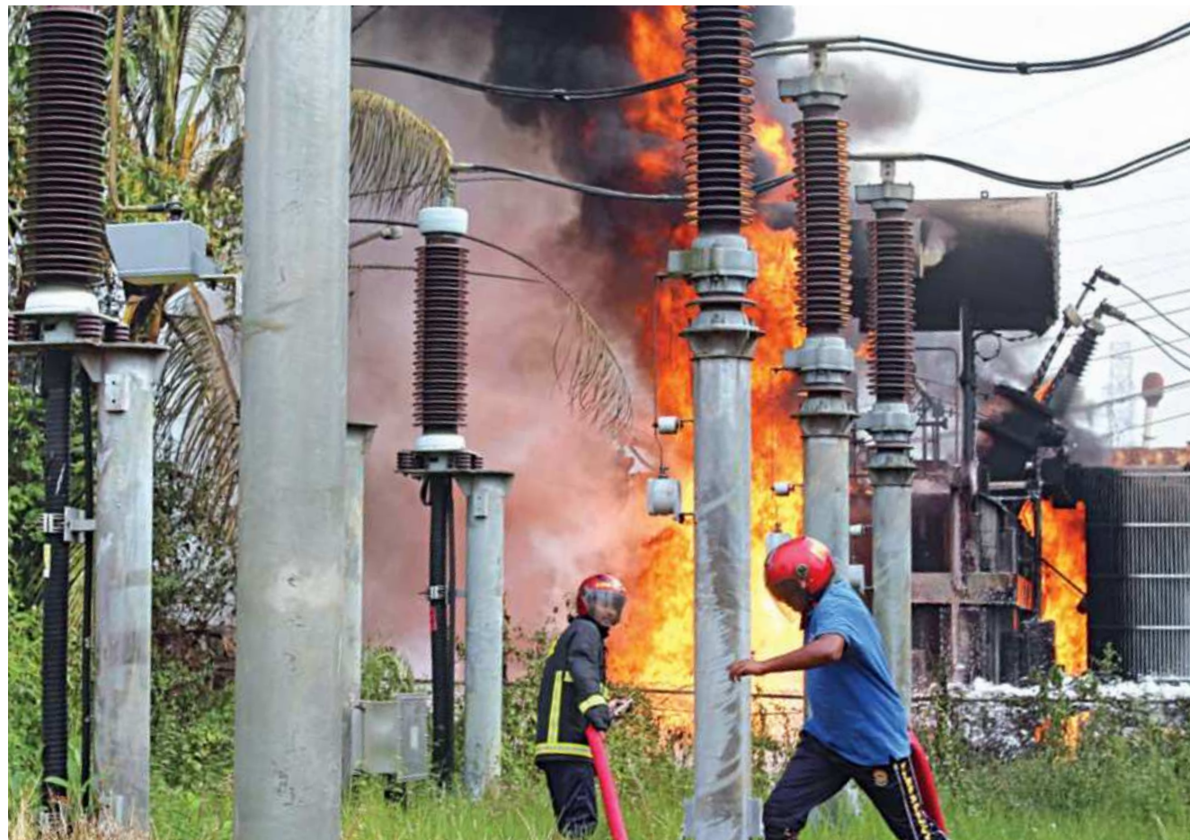
Firefighters fight a blaze at Kumargaon Bidyut Kendra on the outskirts of Sylhet city yesterday morning. The districts of Sylhet and Sunamganj went dark due to the fire which was suspected to have originated from a transformer. The authorities could restore power supply to only a few areas in Sunamganj until last evening.
