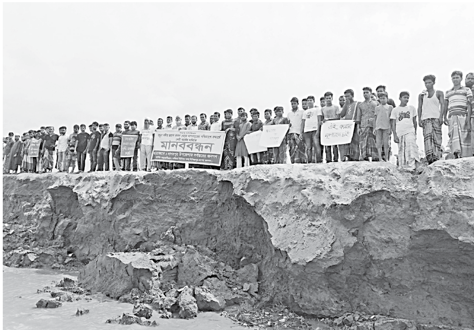
Local people in Solimabad and Doptior unions of Tangail's Nagarpur upazila formed a human chain beside the Jamuna river in Nishcintapur area last week, demanding to construct an embankment in the area to save the localities from erosion.
