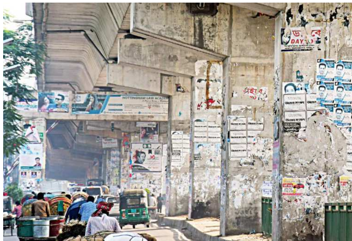
The towering pillars of Moghbazar-Tejgaon flyover are covered with posters to advertise all sorts of stuff, from films and rentals to educational institutes and medical clinics. And as days go by, these pieces of paper degrade or get torn off, but what stays is the unappealing sight for residents and passers-by to witness.
