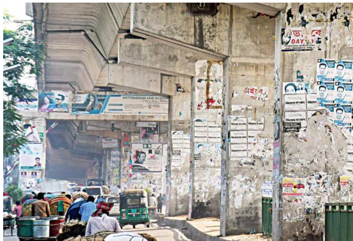
The towering pillars of Moghbazar-Tejgaon flyover are covered with posters to advertise all sorts of stuff, from films and rentals to educational institutes and medical clinics. And as days go by, these pieces of paper degrade or get torn off, but what stays is the unappealing sight for residents and passers-by to witness.
