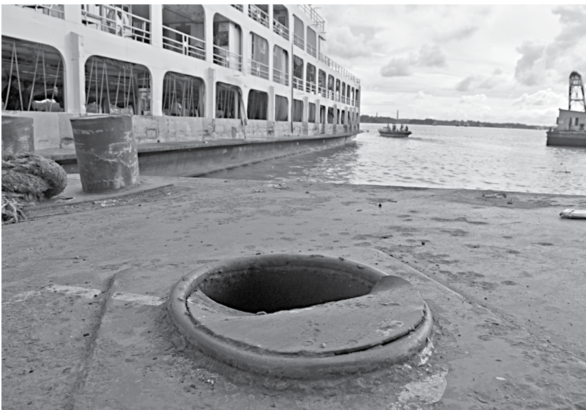
Several spots on Barishal river port's pontoon has been damaged, leading to the creation of potholes. This creates huge risks for passengers -- especially for those with movement handicaps -- who use the area to board Dhaka-Barishal river route launches. This photo was taken yesterday.
