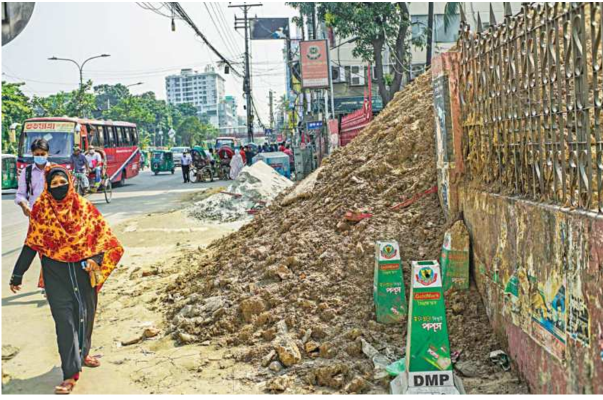
Heaps of soil are spilling out from the capital's Mohammadpur fire station, as authorities are constructing a new building there. The displaced earth has remained in front of the gate and on the footpath for a while now, forcing pedestrians to circumvent the obstacles. This photo was taken yesterday.
