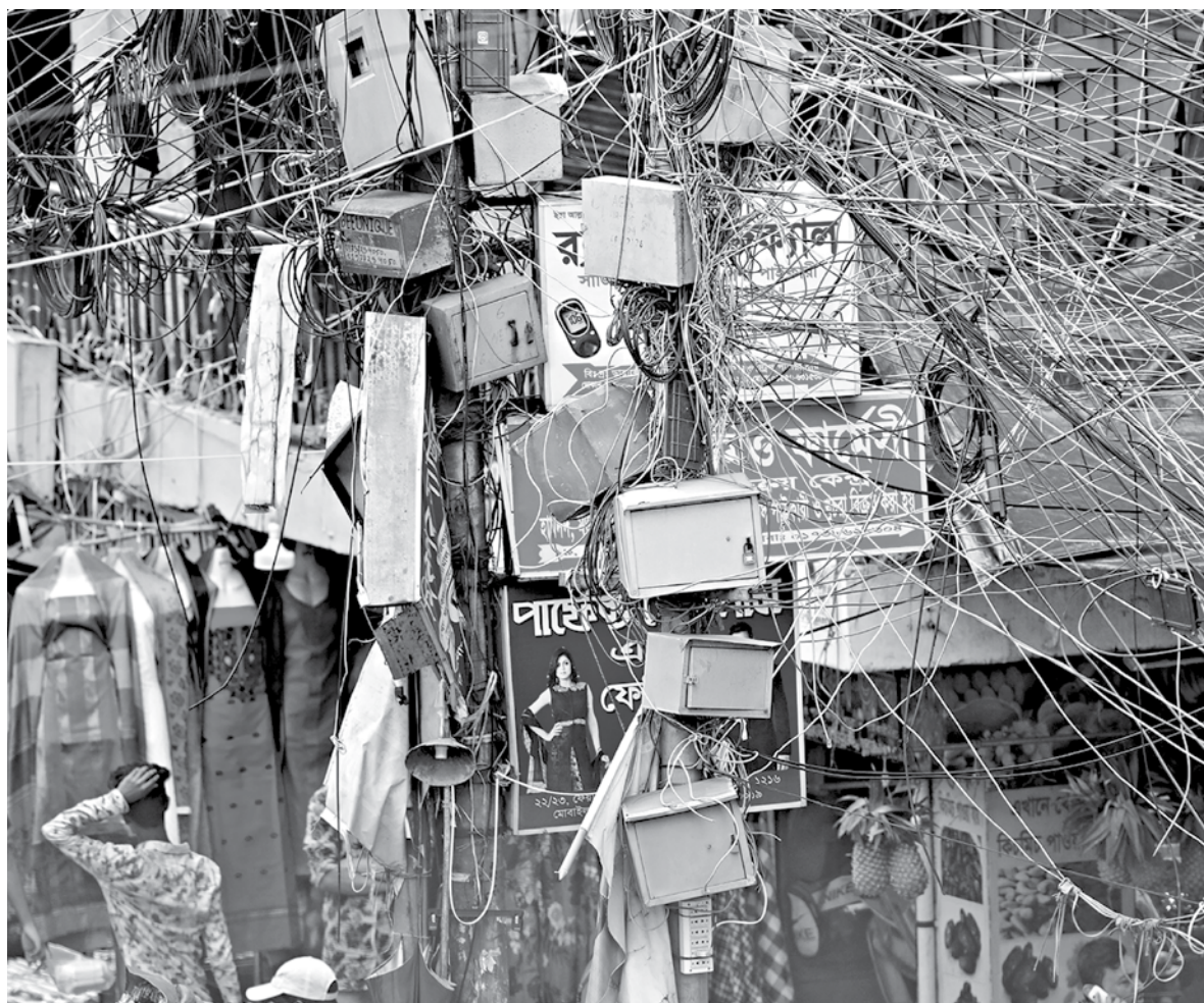
Wires put up by internet service providers are cluttering the capital city's line of sight. Hung from electrical and telephone poles, they cling together and gather dust, while compounding the chance for accidents. This photo was taken yesterday from Mirpur-1.
