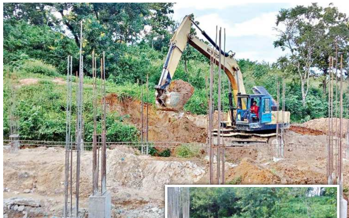
Environmentalists photographed this excavator reportedly razing a part of "Thackeray Tila" of MC College campus on October 11. Days later, on October 25, the same area was seen reshaped to its original state, as if nothing happened. But the soil was still loose.
