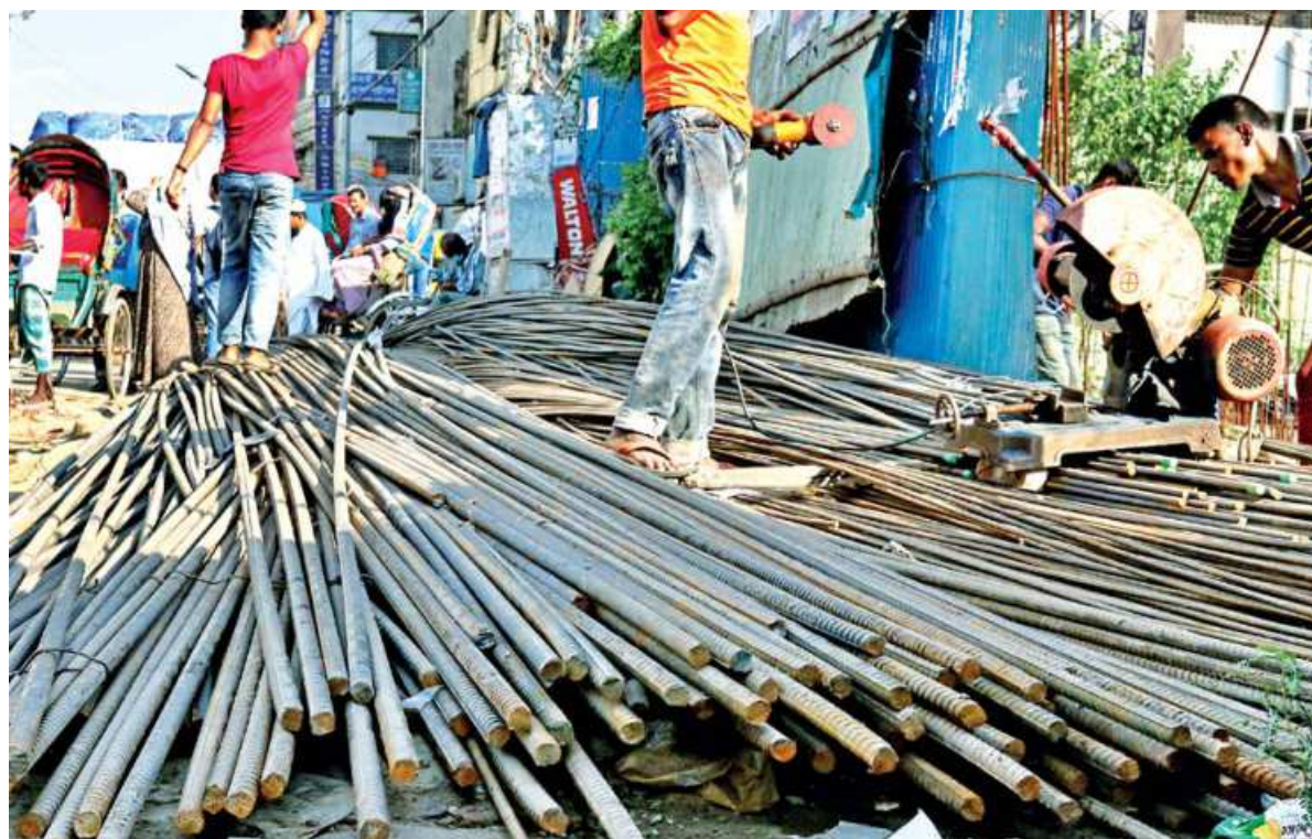
Heaps of iron rod occupy a pavement near the capital's Chankarpool intersection. The rods, being used for the construction of a high-rise, have been kept there for more than a month, putting pedestrians at risk of injuries. The photo was taken yesterday.
