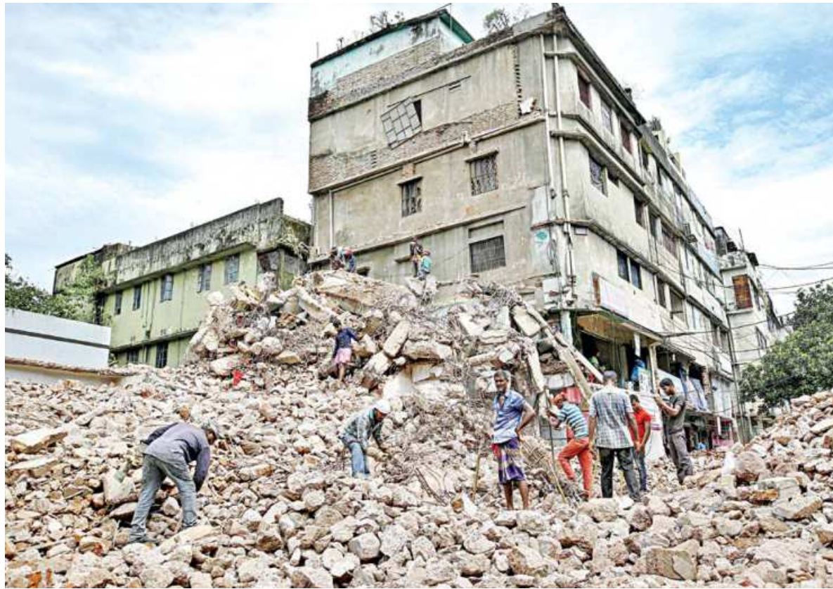
Chattogram Development Authority is demolishing some buildings at Muradpur to make way for canals. Work of canal re-excavation, expansion, renovation, and development is going on to ease waterlogging in Chattogram city. This photo was taken yesterday.
