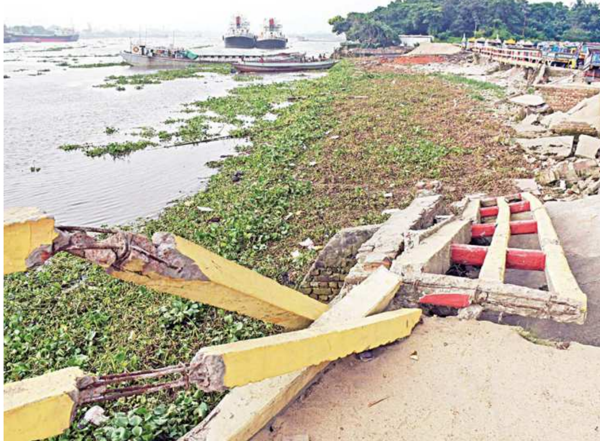
This walkway on the bank of Buriganga River at Munshikhola of Dhaka's Shampur remains in ruins. The structure couldn't bear the load of parked trucks and eventually fell apart, and authorities haven't taken any steps to fix it yet. The photo was taken earlier this week.
