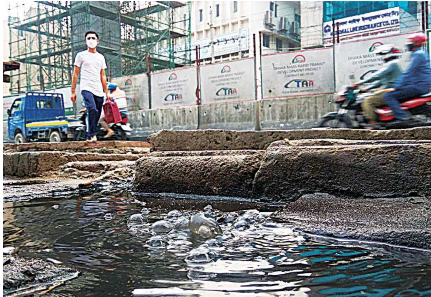
Gas bubbles in open sewer-water in Karwan Bazar. Locals allege that gas has been leaking there for over a year. They informed Titas gas authorities about the leak at different times, but to no avail. The Titas headquarters in only a few buildings away. Recently, a gas leak explosion killed around 30 people in Narayanganj.
