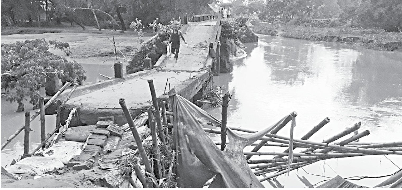
The broken bridge at Baghpara village in Mymensingh's Dhobaura upazila
