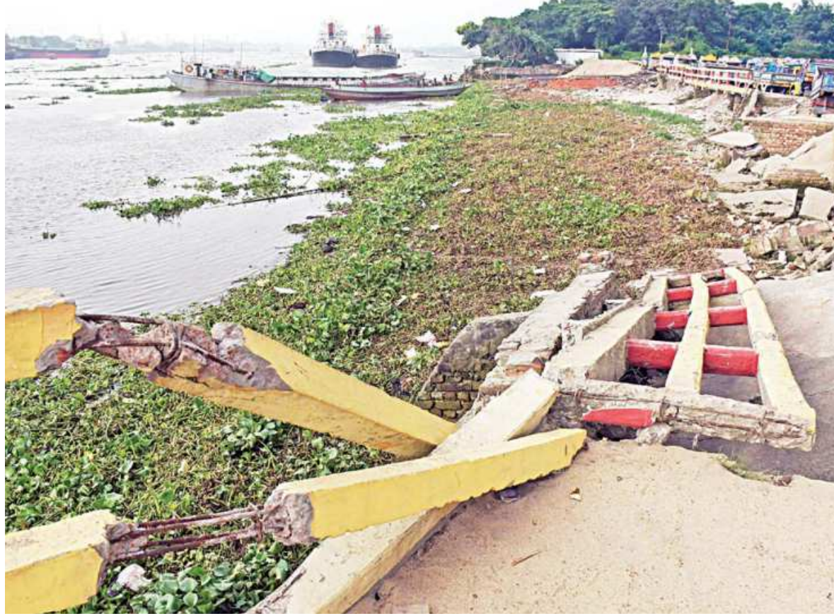
This walkway on the bank of Buriganga River at Munshikhola of Dhaka's Shampur remains in ruins. The structure couldn't bear the load of parked trucks and eventually fell apart, and authorities haven't taken any steps to fix it yet. The photo was taken earlier this week.
