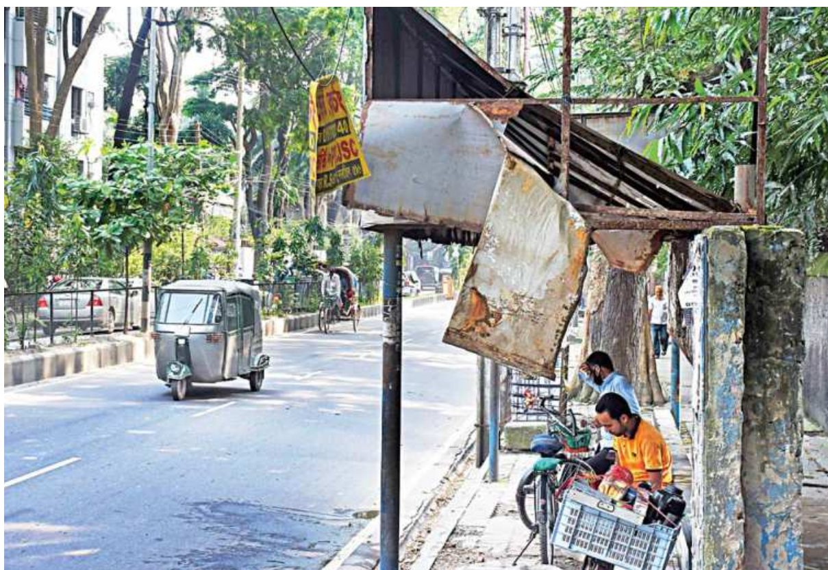
A bus-waiting shed on Asad Avenue stands badly damaged by the elements. Authorities seem least bothered about its upkeep though passengers complain about having to get wet in the rain while waiting for transport there. The photo was taken yesterday.
