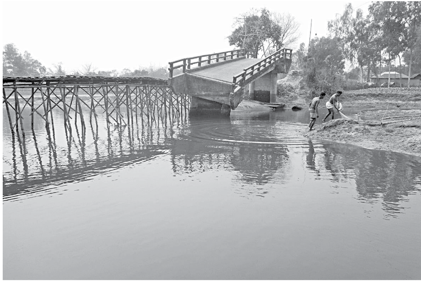
This important bridge, situated between two upazilas of Nilphamari and Dinajpur, over Bhulli river in Nilphamari Sadar upazila has been lying unrepared since it collapsed in 2017. The photo was taken recently.
