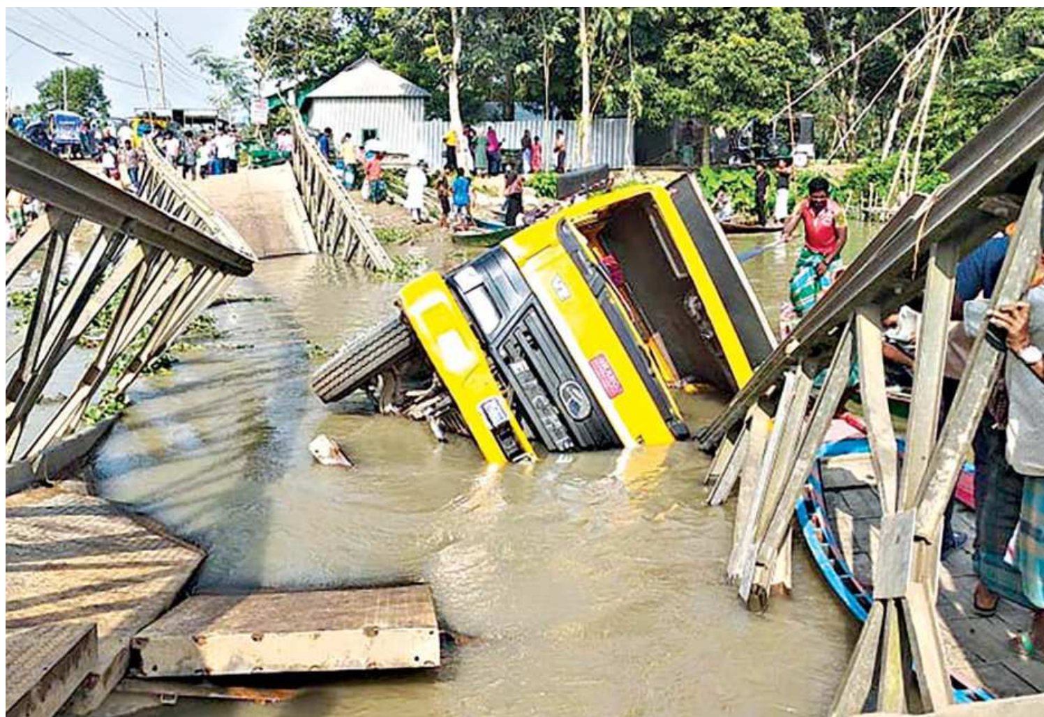
A bailey bridge over Langulia river on the Tangail-Basail road at Nakasim area collapsed on Sunday after a sand-laden truck got on it. With the vehicle falling into the river along with the collapsed bridge, direct road communications to Basail and Sakhipur upazila from Tangail town were disrupted.
