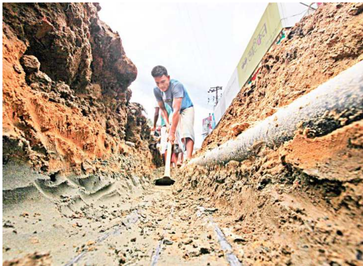
Within three weeks after it was last dug for underground electrical and water works, Sylhet's Chowhatta-Zindabazar road is being dug into again. City corporation sources said contractors for previous projects did not dig it properly, and the new round of digging is a rectification of their faulty delivery. This photo was taken yesterday.
