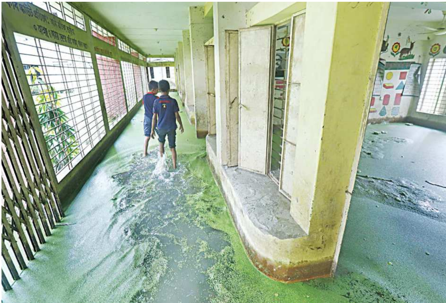
Boys walking ankle-deep in water on the corridor of Kajlpar Government Primary School in the capital's Jatrabari. The severe and prolonged waterlogging is the result of a dysfunctional drainage system in the area. The photo was taken yesterday.
