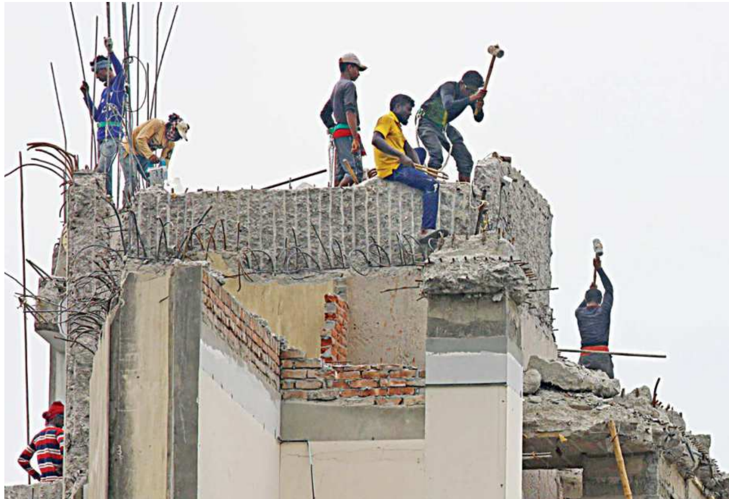
Some of the workers demolishing the illegal BGMEA building have no gear to save them from falling off the high-rise building. Tragedies at construction sites are all too common because of such utter disregard for safety.
