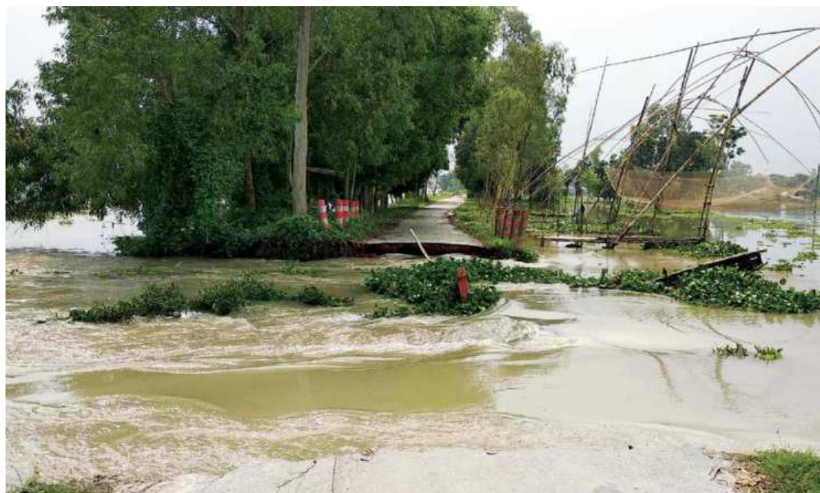
Floodwater devoured a culvert on Basail-Natiapara Road in Tangail's Basail upazila early yesterday, disrupting road communication among 30 villages of Basail and nearby two other upazilas. The photo was taken later in the afternoon.
