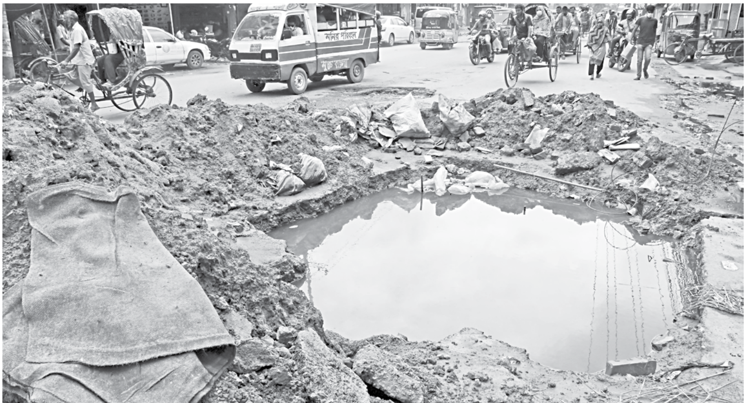
At one point on Mohammadpur's Ring Road in the capital, Dhaka Wasa had dug a large hole for their work two and a half months ago, and the scene hasn't changed since then. As a result, a bottleneck has formed at that point, constricting traffic and pedestrian movement. The photo was taken earlier this week.
