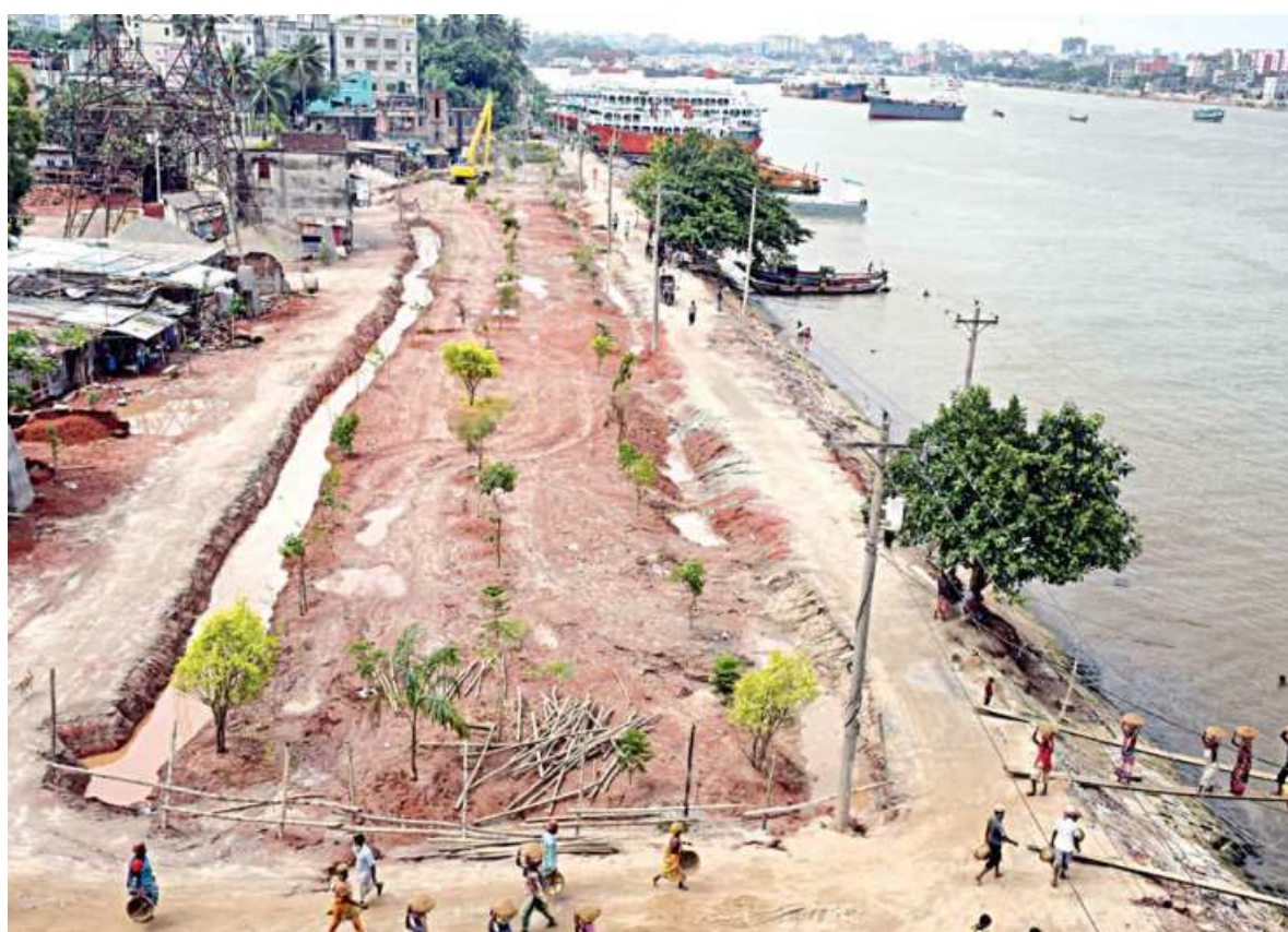
Encroachment has been a perennial problem along the banks of river Buriganga, and many a time the culprits returned to the spot a few months after eviction. Bangladesh Inland Water Transport Authority (BIWTA) recently evicted encroachers from this spot in South Keraniganj, and are now planting trees there in a bid to turn the riverside into a park, and also ensuring it is not taken over again. The photo was taken yesterday.
