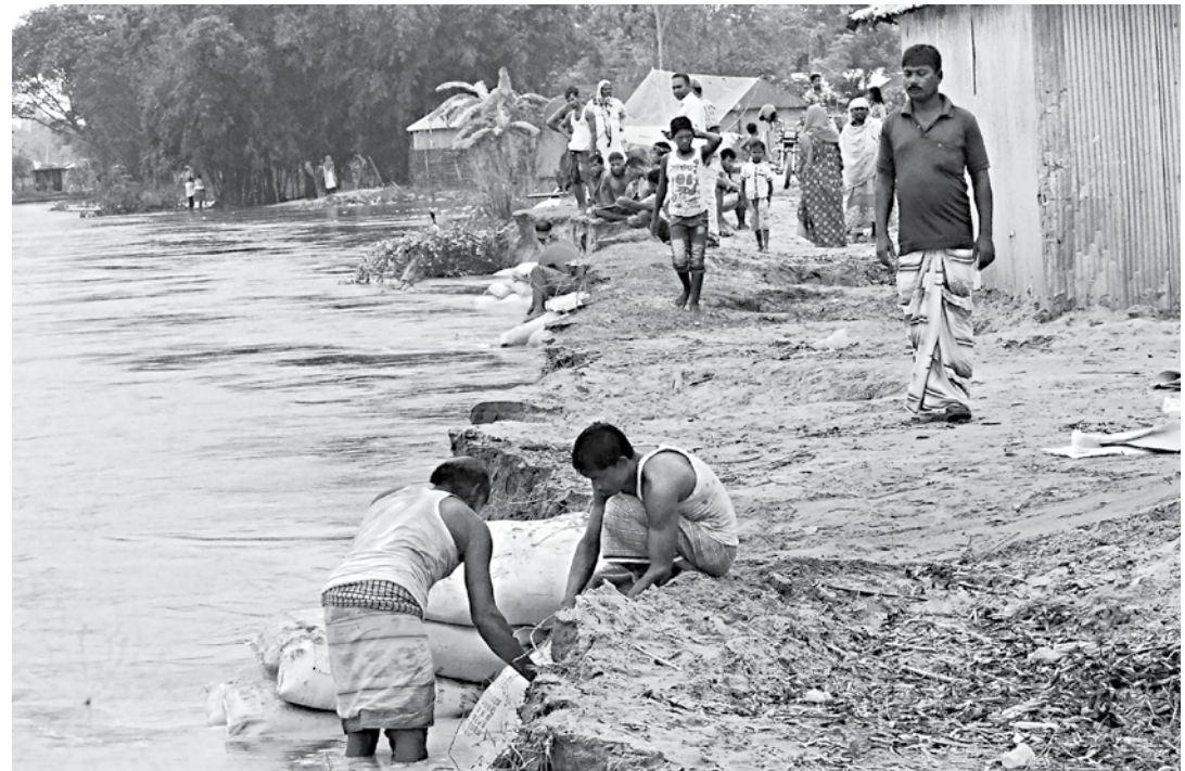
They do not know whether the few sand-filled bags they are placing on the edge of the river will make the aggressive Teesta stop devouring their land. But the inhabitants of Purbo Ichli village in Rangpur's Gangachara upazila have no other choice. PHOTO: KONGKON KARMAKER
