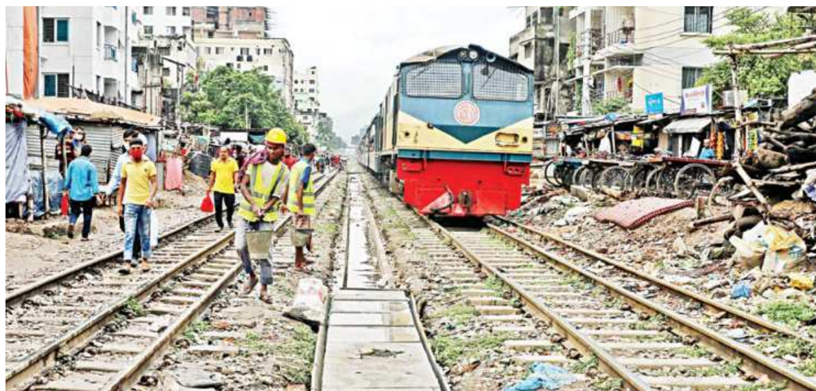
Rail workers installing a drain between the lines near Malibagh Level Crossing in the capital yesterday. This section of the lines has been prone to waterlogging.
