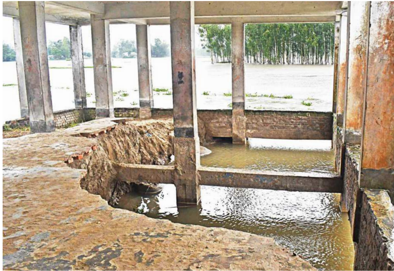
The Char Godagari Government Primary School is sinking into the Bangali river in Bogura's Sariakandi upazila. It is only a matter of time before the school building completed in 2002 is devoured by the river that has been eroding its banks over the last four days.
