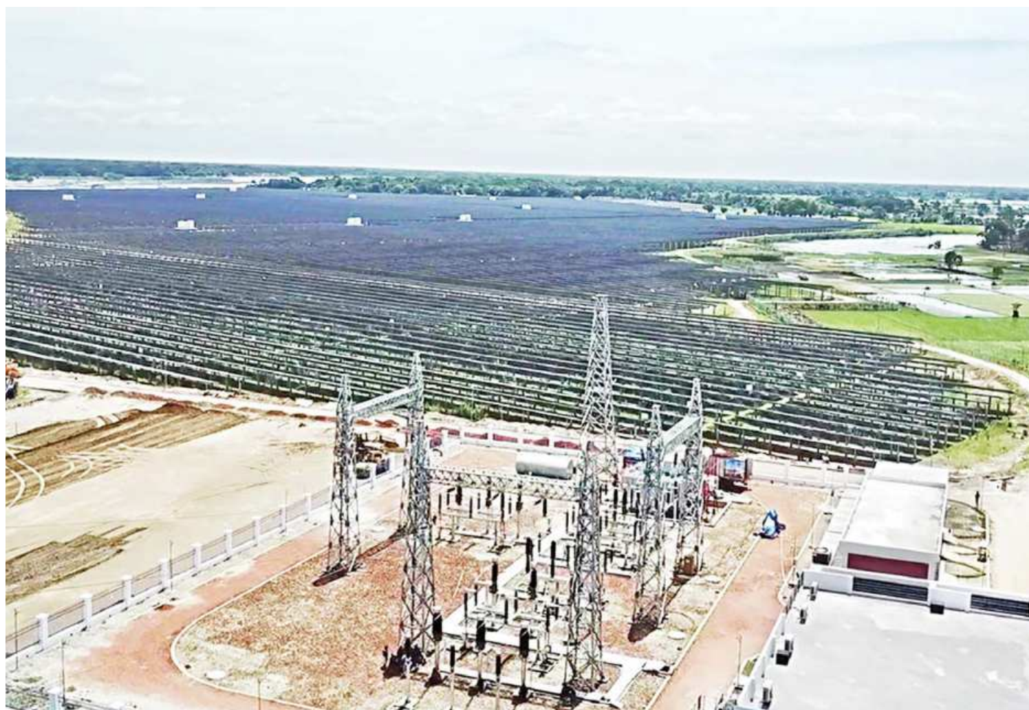
The country's largest solar-based powerplant in Mymensingh's Sutiakhali area is set to start operation in the first week of October. The 50-megawatt plant was established to meet the government's target of using renewable energy to produce 10 percent of the country's total electricity by 2021.
