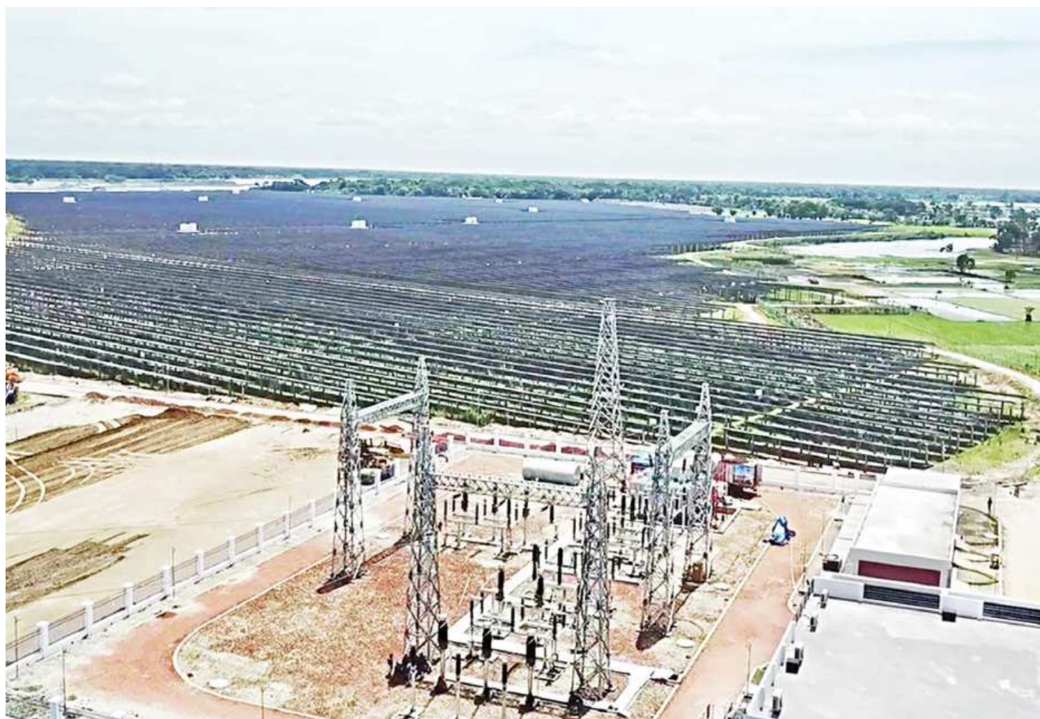
The country's largest solar-based powerplant in Mymensingh's Sutiakhali area is set to start operation in the first week of October. The 50-megawatt plant was established to meet the government's target of using renewable energy to produce 10 percent of the country's total electricity by 2021.
