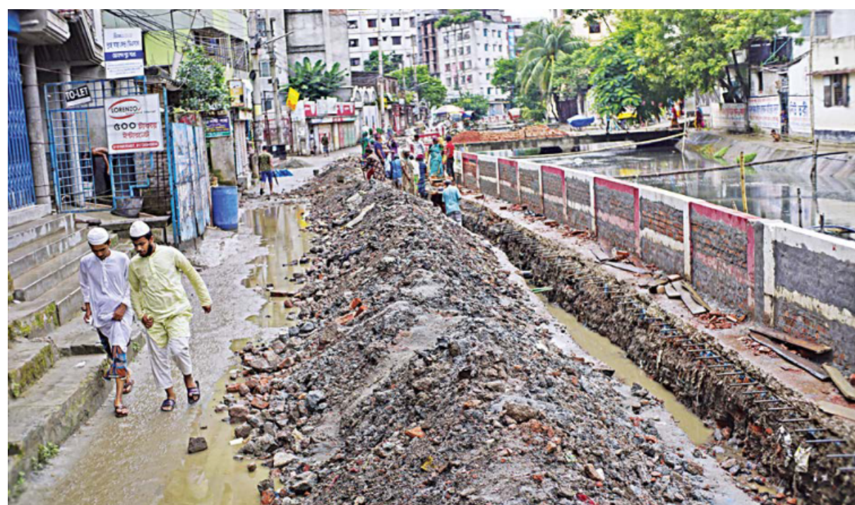
Development work at this two-kilometre road in Mohammadpur -- stretching from Mohammadia Housing all the way to Beribadh -- has been going on for over a month. For more than two weeks, the road has been cordoned off for the works. This is causing immense suffering to the residents of the densely populated area, especially due to the rainfall of the last few days.
