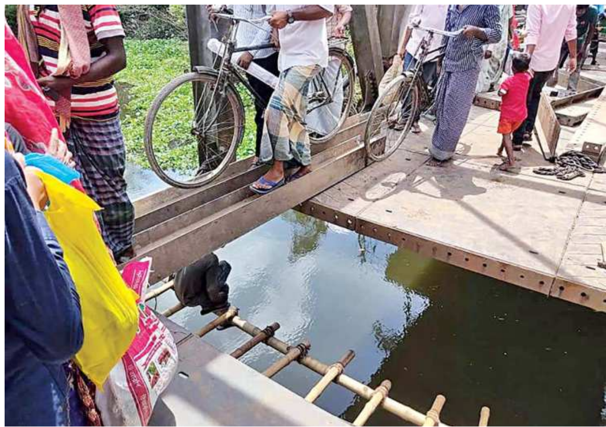
Pedestrians and cyclists undertaking a precarious crossing over a section of a Bailey Bridge being repaired on the Tangail-Aricha regional highway in Tangail's Nagarpur upazila. This photo was taken yesterday.
