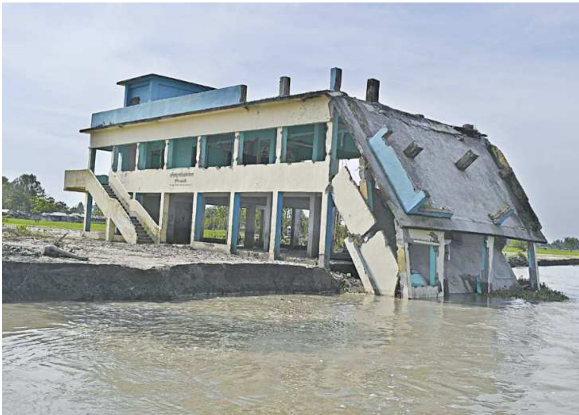
The mighty Jamuna devouring Char Dighapara Government Primary School in Bogura's Sariakandi upazila yesterday. The school building was constructed in FY 2004-5 at a cost of Tk 28 lakh. The authorities said the river was at least two kilometres away from the school building three years ago.
