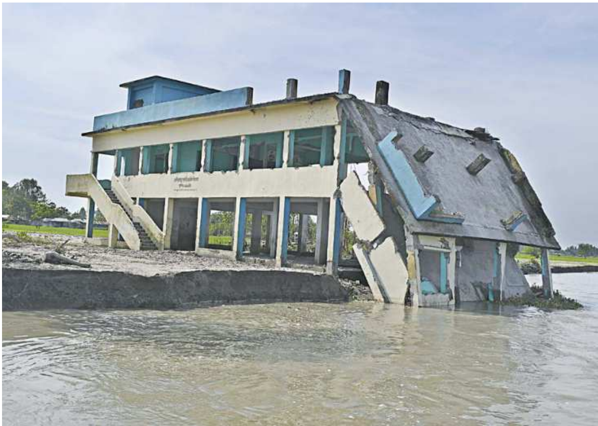
The mighty Jamuna devouring Char Dighapara Government Primary School in Bogura's Sariakandi upazila yesterday. The school building was constructed in FY 2004-5 at a cost of Tk 28 lakh. The authorities said the river was at least two kilometres away from the school building three years ago.
