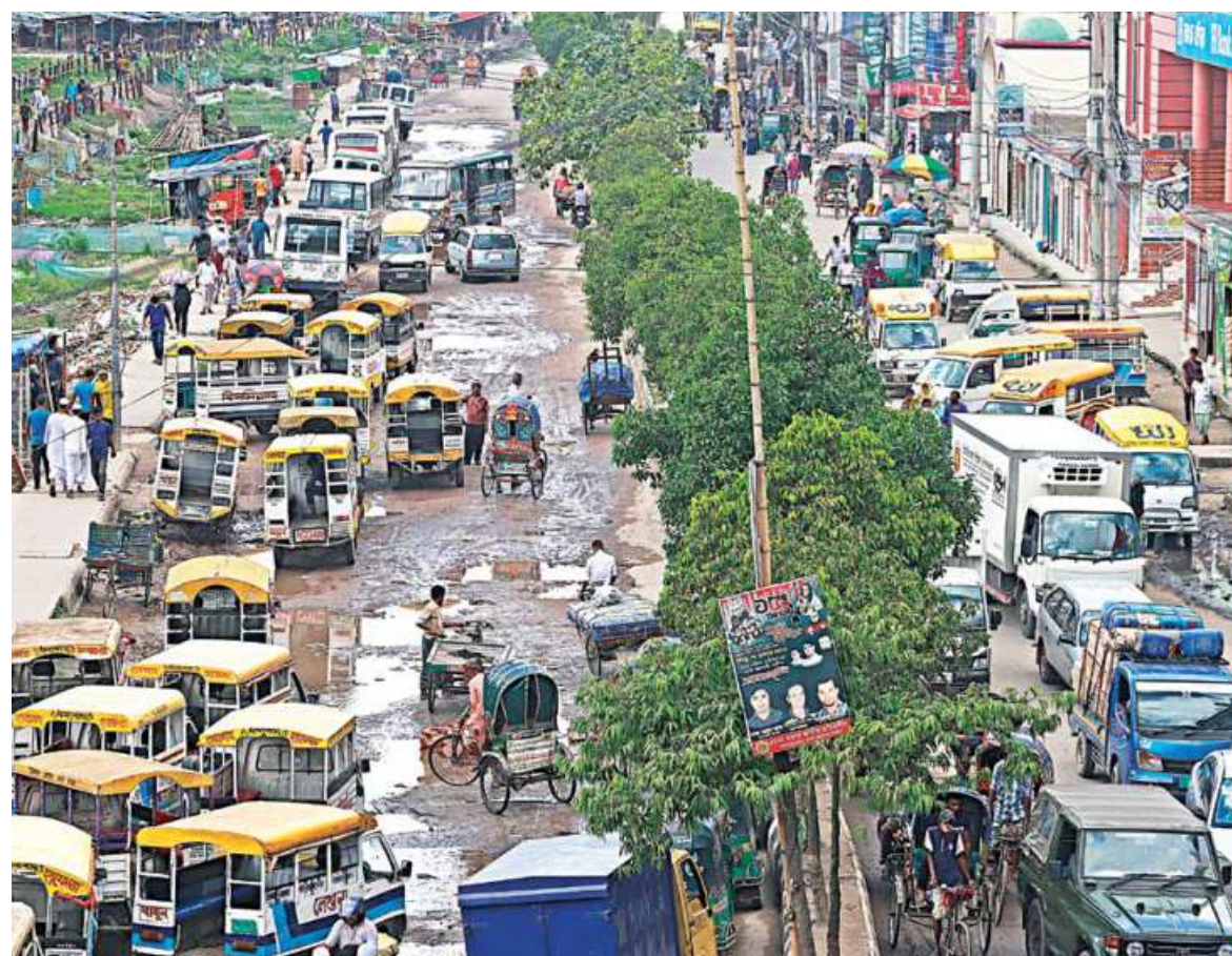
This road in Jurain Railgate area of the capital has become a virtual human hauler stand, and for good reason too. The dilapidated carpeting on the road with puddles all over has left it unfit for vehicular movement. Locals say the situation has been like this for a long time.
