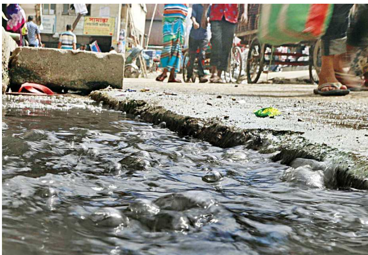
Gas bubbles forming in this roadside drain near Alam Market in the capital's Jurain. A gas line runs parallel to this drain and the leaking gas has created an overpowering odour, but no action is being taken despite complaints from locals. This photo was taken on Saturday.
