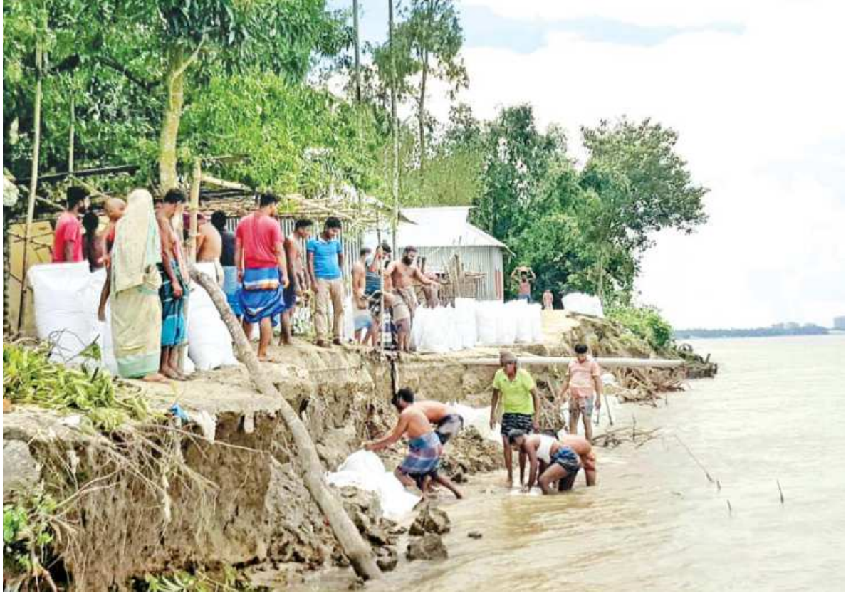
Villagers dumping sacks of dirt to save their locality from the mighty Jamuna. Erosion began in the different parts of Tangail as the river's water level started to drop. This photo was taken at Bhuapur's Bhalkutia on Saturday.
