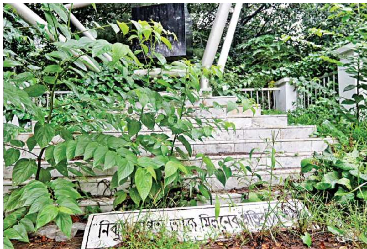
The Milon Smriti Stamba in TSC area of Dhaka University is in a bad shape due to a lack of maintenance. The memorial was built to commemorate Dr Shamsul Alam Khan Milon, who was killed by thugs at the height of the anti-autocracy movement in 1990. The physician's supreme sacrifice had transformed the movement into a mass upsurge that prompted the fall of the then autocratic regime of HM Ershad. The photo was taken yesterday.
