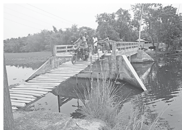
This bridge, built on Chandrakura Canal in Nilphamari Sadar upazila about a year ago, is unusable for commuters due to the lack of approach roads.
