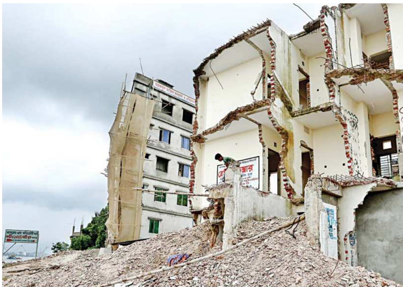
Using a hammer, a worker demolishes a part of a building in Kholamora Munshihaat area of the capital's Kamrangirchar yesterday. The building's owner hired workers for the work as the BIWTA was carrying out a drive in the area to remove illegal structures from the Buriganga. The owner said part of his building was legal and that he feared the BIWTA might demolish the entire building.
